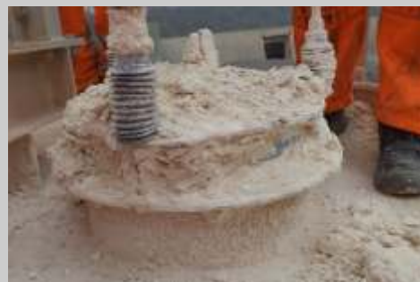
Pressure relief valves (PRV) are the last line of defence against over-pressure. With effective protection and servicing, blocks like the example above can be avoided.
