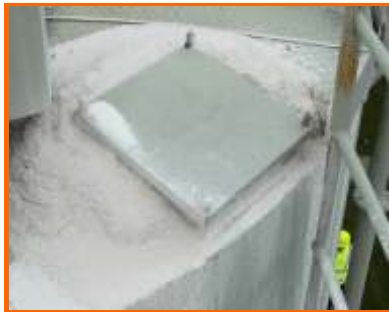
Product discharge from the PRV
