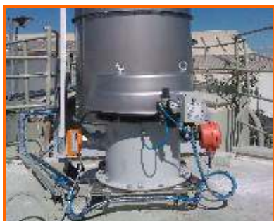
Latest testable silo instruments
