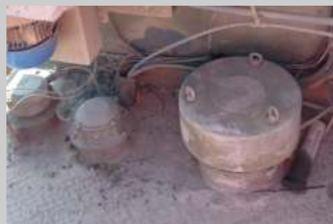
After physical testing, this PRV and pressure sensor failed to operate at the correct set points. Previously this was serviced with only a visual inspection!
