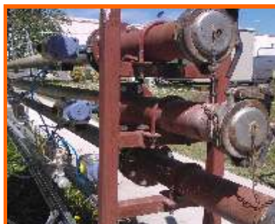
Valves fitted for auto shut-off
