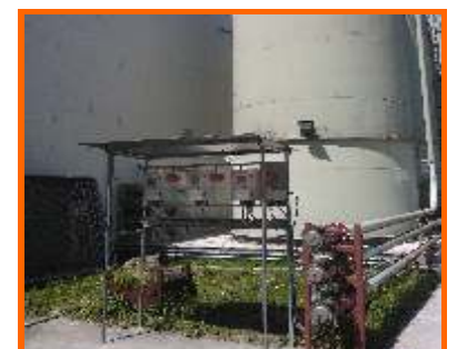
Display and control at fill point
