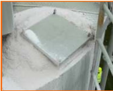
Product discharge from the PRV
