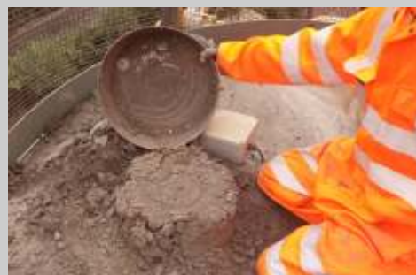
This PRV appeared fine, but an inspection under the lid reveals the opposite. This problem would indicate the silo safety system has totally failed!
