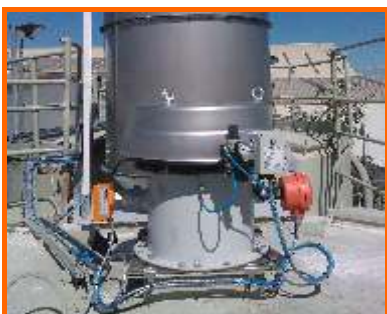
Latest testable silo instruments
