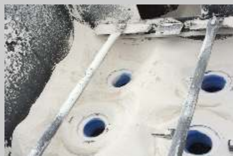
Damaged and neglected filter cartridges will cause emission issues if they burst, or if they are completely blocked they have the potential to cause serious silo damage!
